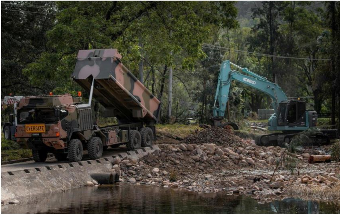
An Army HX77 and excavator being used to reconstruct a bridge near Wauchope, NSW, which was damaged by the floods. Photo: Private Jacob Hilton
